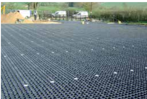
A permeable parking area is made from recycled silage wrap. The car park is sown with low-growing flowering herbage to attract insects and bees.
