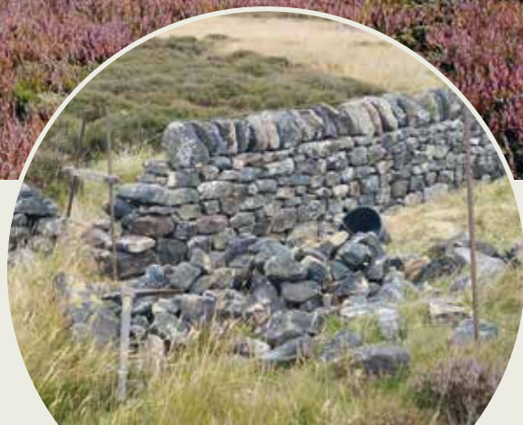
One of the many stone walls being repaired on Geoff's grouse moor
