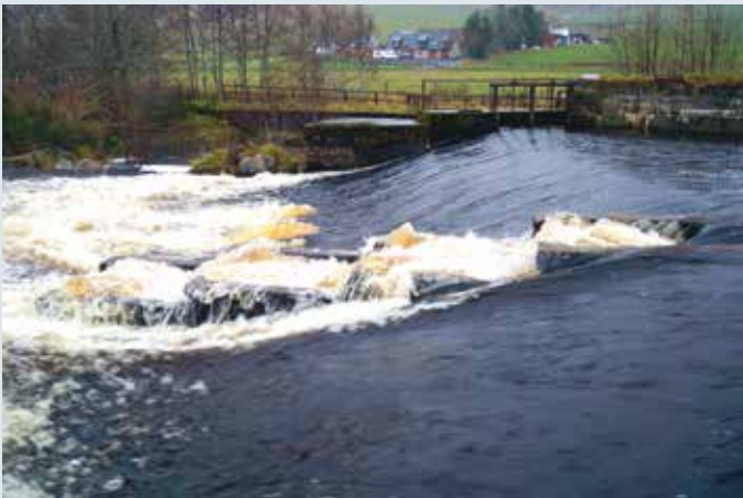
The old concrete fish ladder is to be replaced to help salmon migration
