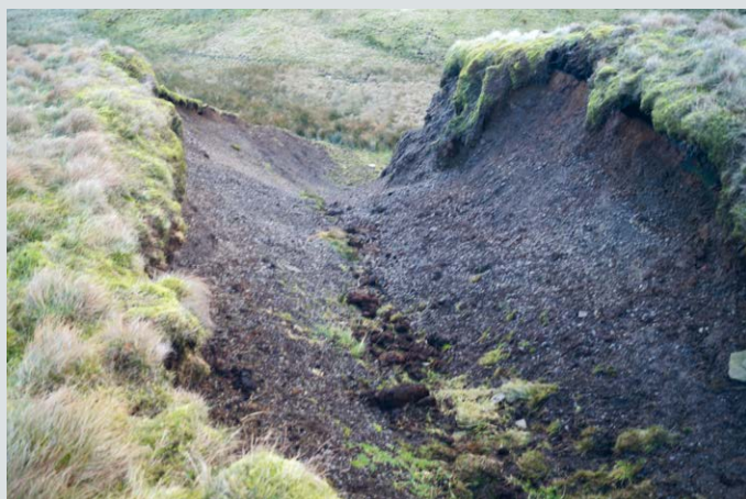
Drains or grips can cause erosion, which colours the drinking water.
